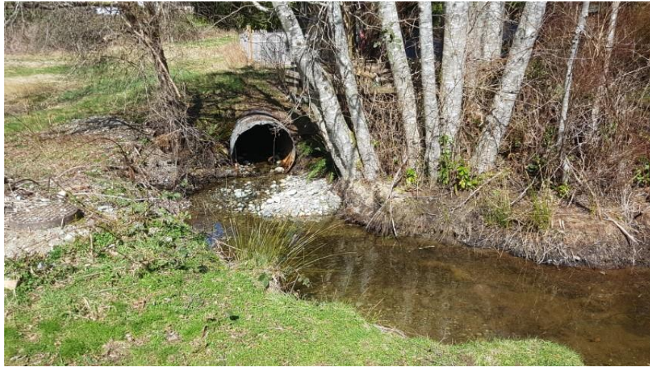
Photo 13 - Creek 3C outlet pipe at H'Kusum Park. Note pile of dredged gravels on left side of ditch.
