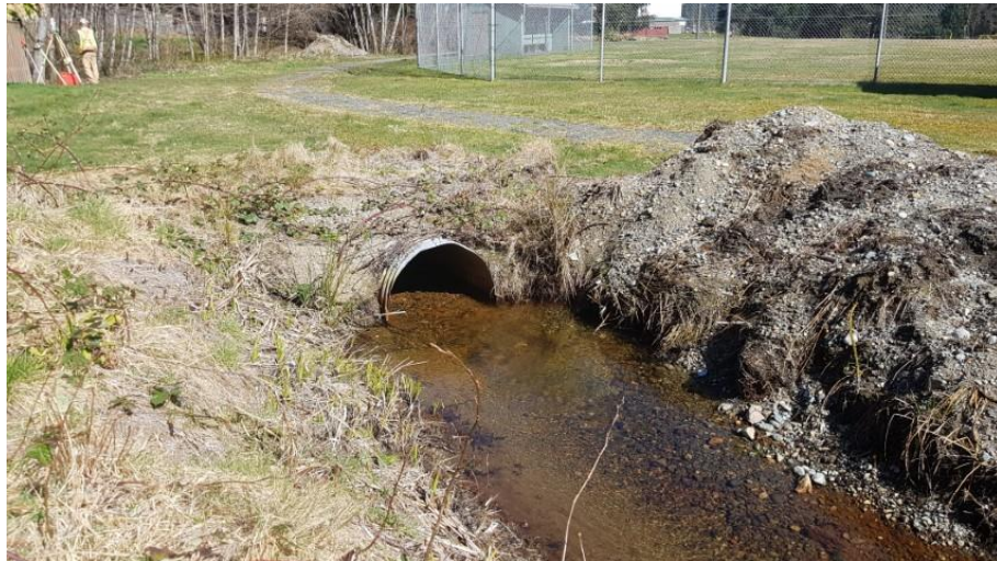
Photo 8 - Creek 3A & 3B outlet in H'Kusum Park. Note gravel depth in pipe and ditch, and pile of dredged material next to ditch.
