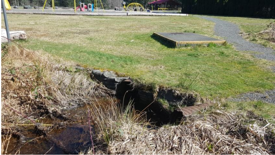
Photo 9 - 600mm CSP pipe inlet to DMH 2
