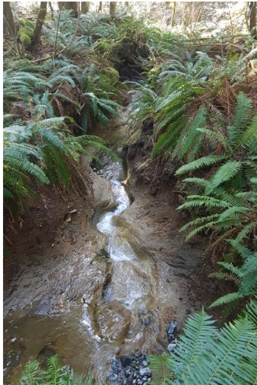
Photo 6 - Creek 3A & 3B drainage channel below wooden log diversion structure. Note exposed gravels in walls and continued erosion in bottom of channel
